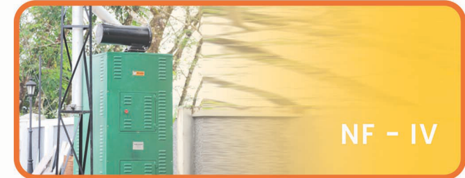
INCINERATOR NF - IV
